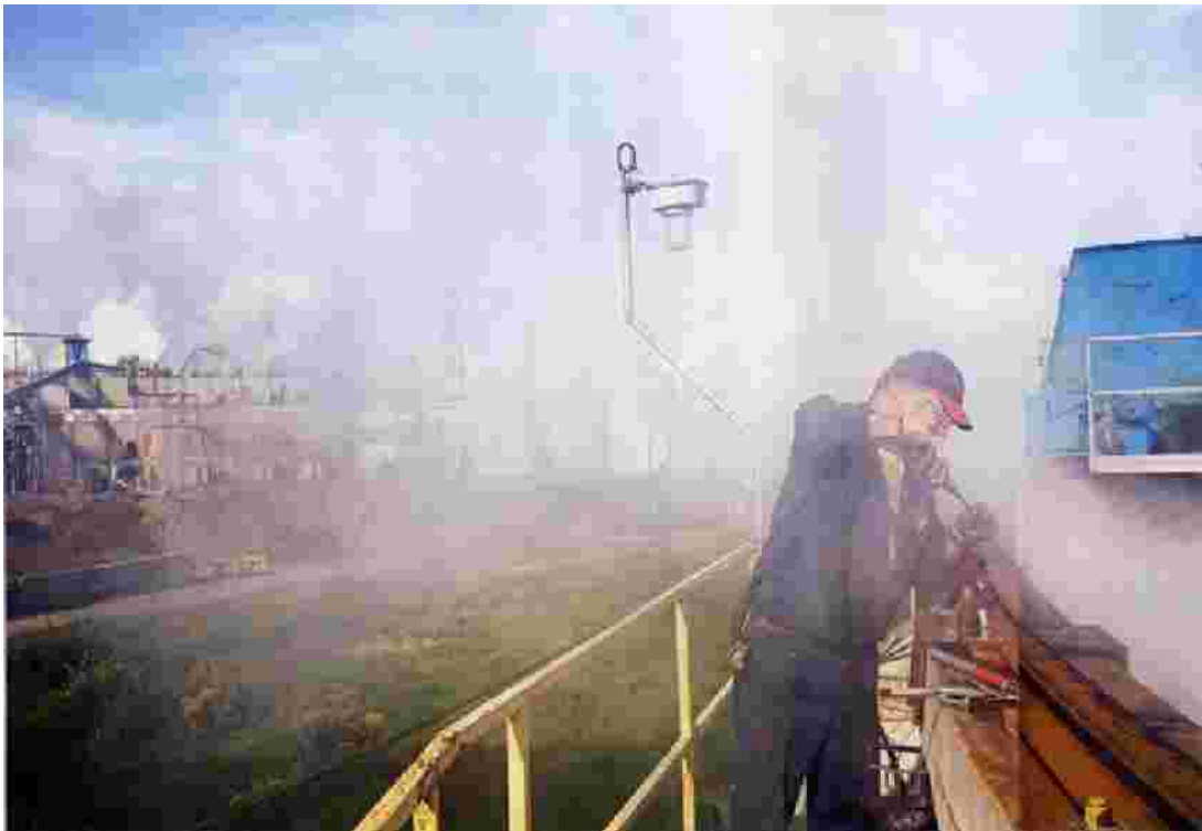
Guy Jalbert repairs the rail of a wastewater treatment tank at the Kruger
